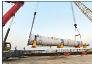
650 Ton Crane and 450 Ton Crane in a tandem lifting operation offloading Column weighing 170tons
